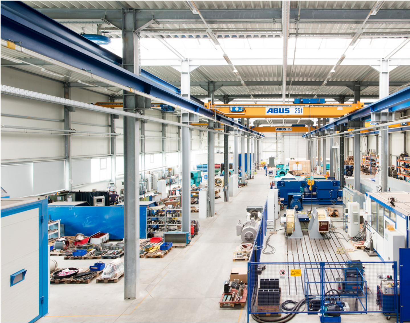
Test field for electrical motors and generators up to 11 kV.
