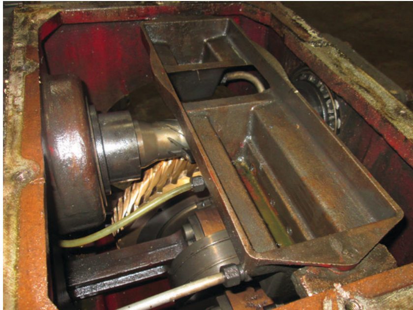
Fig 2. The pump internals were badly worn.
